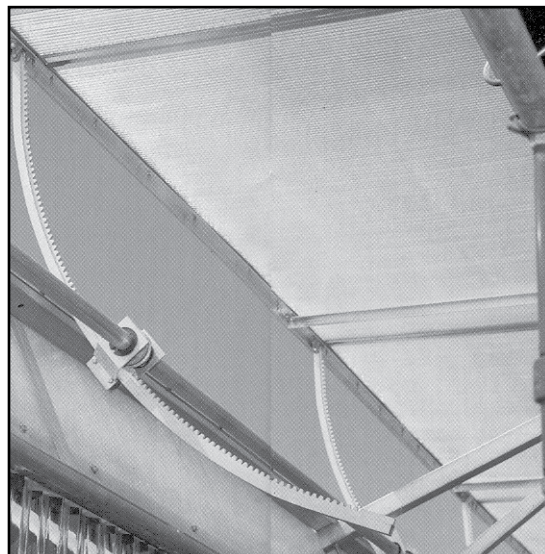
CURVED POWERRACK™ MOUNTED ON GREENHOUSE WITH VENT IN A PARTIALLY OPENED POSITION.
